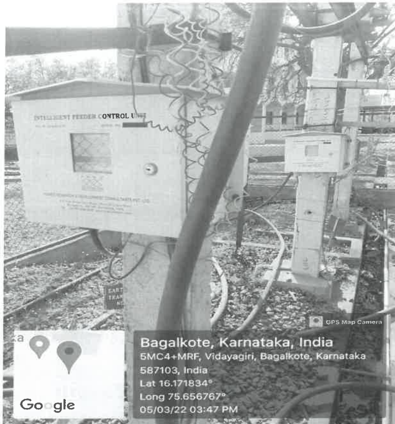
Fig.6: Intelligent Feeder Control Unit at DTC of BEC SCADA
