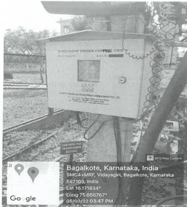
Fig.5: Intelligent Feeder Control Unit at DTC of BEC SCADA
